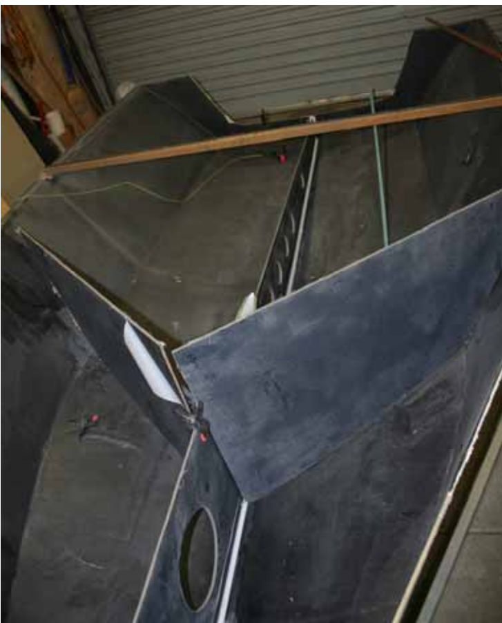
Below: Simon Blatchford's partly finished new hull with the bulkhead fitted and first longitudinal frame fitted and bonded. Flat panels make for easy construction. High res views one , two and three here.
